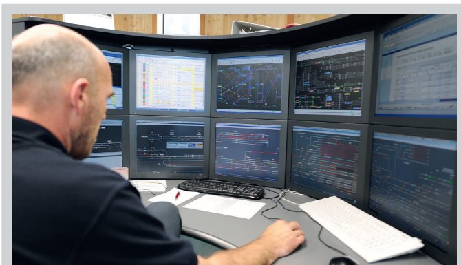
Figure 1: Control centre – track vacancy detection is the most important application for wheel detection
